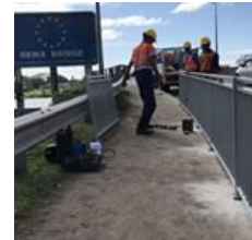
Railing works begin at the new Rewa Bridge! Fulton Hogan staff at work! #keepingourchildrensafe #Nausori #RewaTailevuNaitasiri
